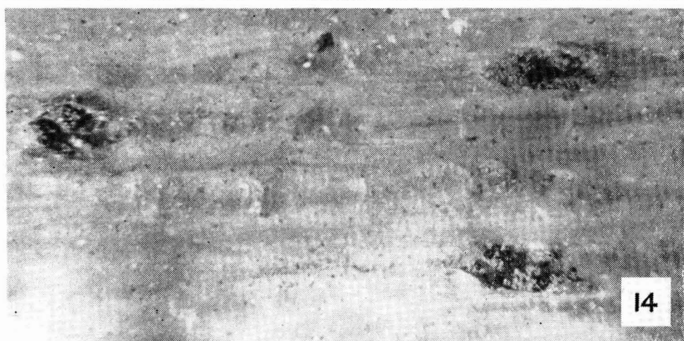
FIG. 12. TYPICAL VARNISH FAILURE ON WOOD AFTER WEATHERING
