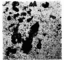
22 months' exposure—extensive flaking is the result when Emulsion Paint does not contain Mica.
