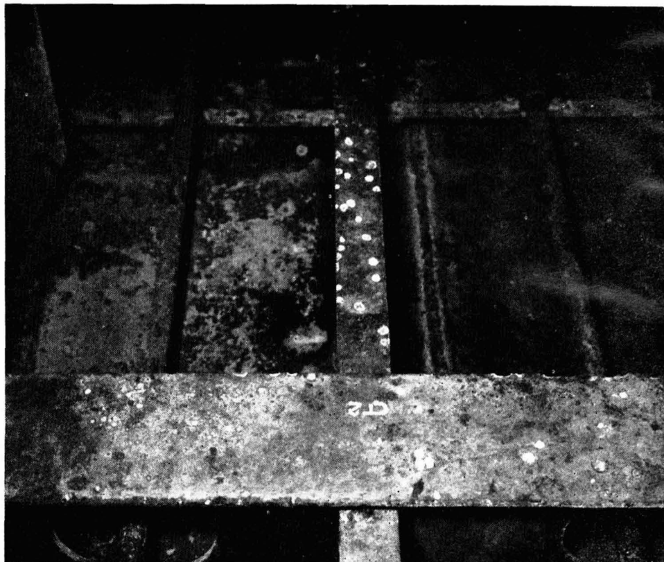
Fig. 1. Examples of pit corrosion
