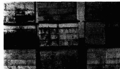
Fig. 3. Algal growth on painted miniature walls. The walls were exposed at ground level, but were rearranged for photographing
