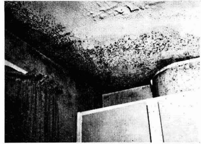
Fig. 4. Mould growth resulting from condensation
