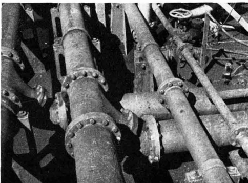
Fig. 8. Pipework in the manifold area, illustrating the difficulties facing maintenance teams
