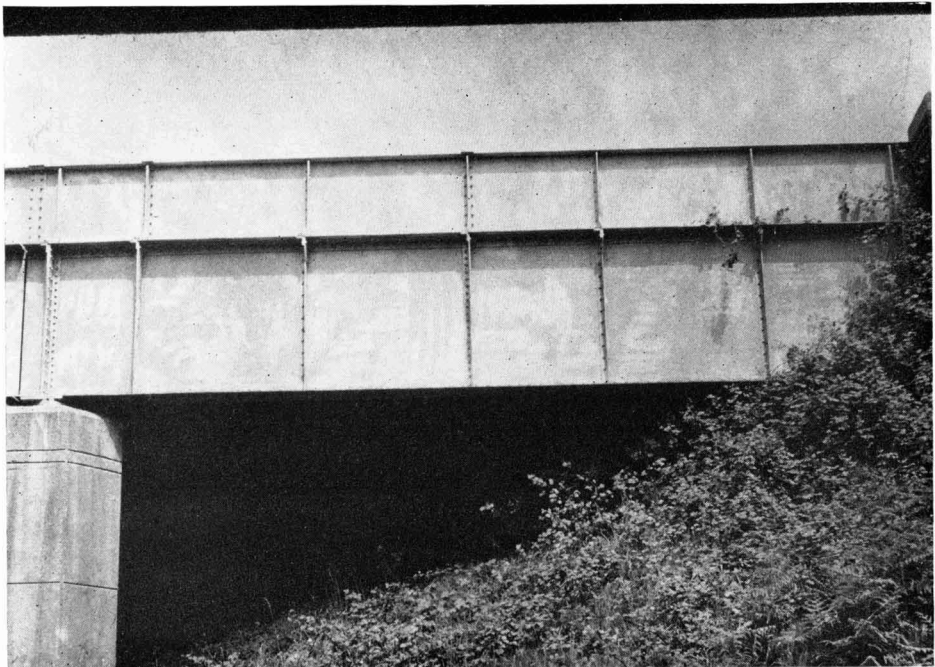
Fig. 2. Typical erosion of white lead paint BS2525 during 10-15 years of exposure in mild industrial conditions. Patches of the primer are beginning to become visible
