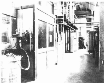
The wall mounted Graco Monark delivers the primer to the booth. The air powered agitator is mounted on the drum cover.
