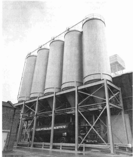
Installation by Portasilos of five 64 tonne capacity Cellulose Acetate silos, mounted on vehicle access structures, at the Lancaster plant of Nelsons Acetate Ltd.
