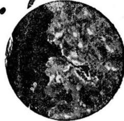
Sectional view of a masonry surface showing the porous condition due to weather erosion.
