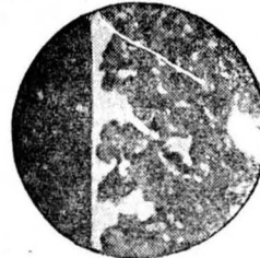
The final coat leaves a clean flat finish and has rendered the surface absolutely watertight and non-porous.
